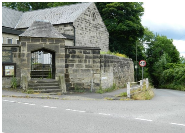
Now re-pointed in cement mortar but probably lime in the first instance
