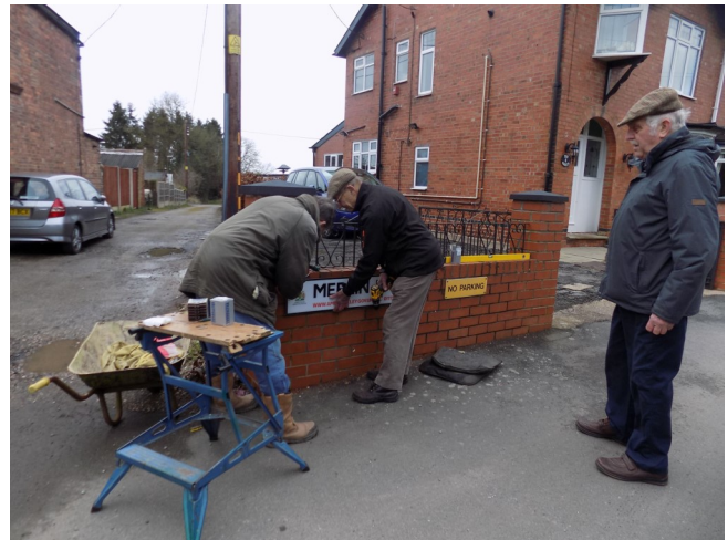
Michael and Ron Harrison fixing the new road nameplate. Alan Tunstall, who first suggested the name Merlin Lane, is supervising
